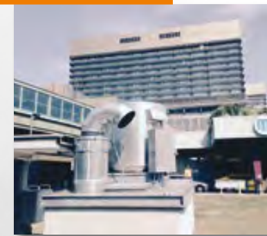
Smoke exhaust fan, Vienna General Hospital.
