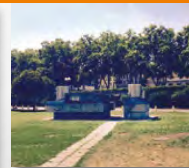
Smoke exhaust fans on the open area above Vienna General Hospital underground car park.
