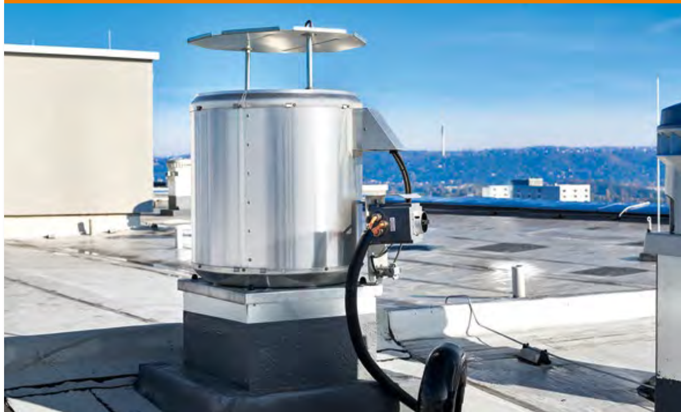
Three bus cables are plenty: one power supply for the switch cabinet, one power supply for the smoke exhaust fan and one communication cable for the TRGX X-FANS BVD 315 smoke exhaust fan on the roof of the high-rise residential buildings in Dresden-Prohlis.
