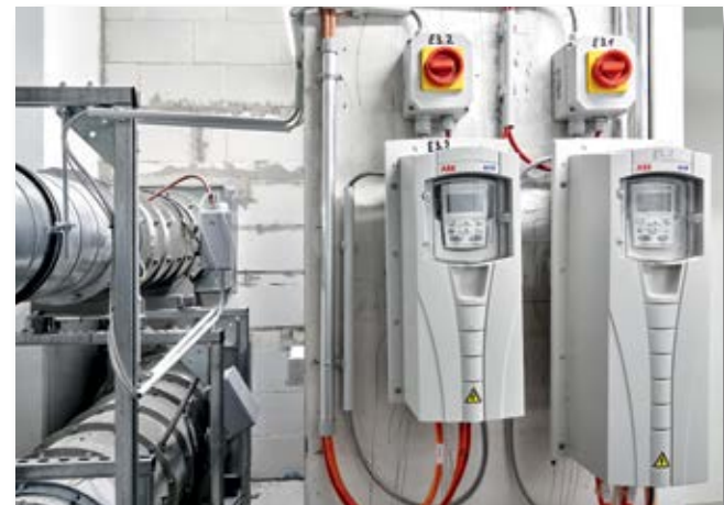
Frequency inverters make speed adjustment of smoke exhaust fans possible
